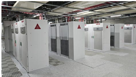
Suwon DC UPS
