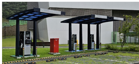
Chuncheon DC EV Charging Stations
