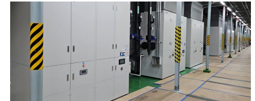
Suwon DC temperature and humidity chamber
